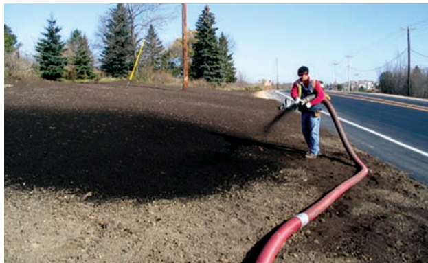
GIVING IT BACK TO NATURE: COMPOST BEING USED ON A HENNEPIN COUNTY ROAD CONSTRUCTION PROJECT IN EDEN PRAIRIE.
